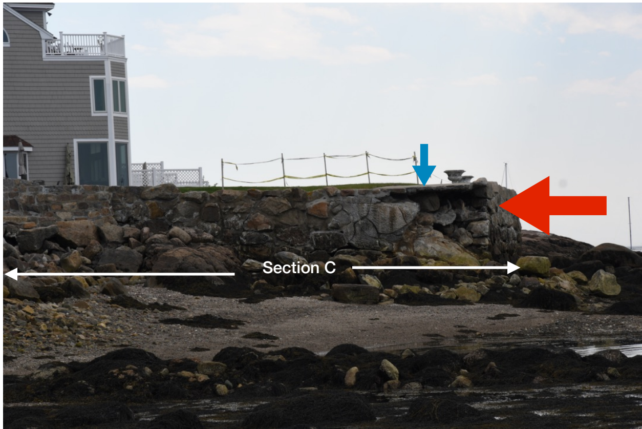
view of section C showing the failed corner just below the two urns
